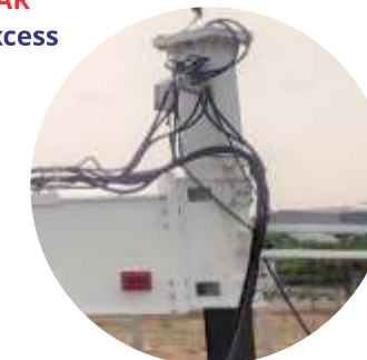
ONE CONTROL BOX with emergency switch on each leg
