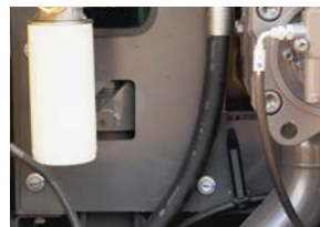
Baffle Plate between engine & pump compartment
