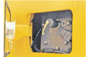
Battery cut-off switch
