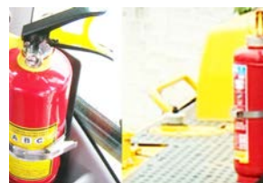
Manual Fire Extinguisher (Inside / Outside the Cab)
