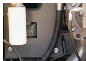
Baffle Plate between engine & pump compartment
